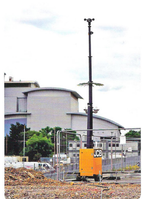
CCTV systems can prevent theft and pilferage.
